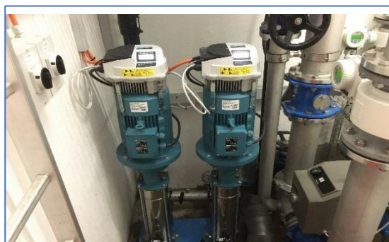
Pumpen Reservoir Chilenwald 2020
